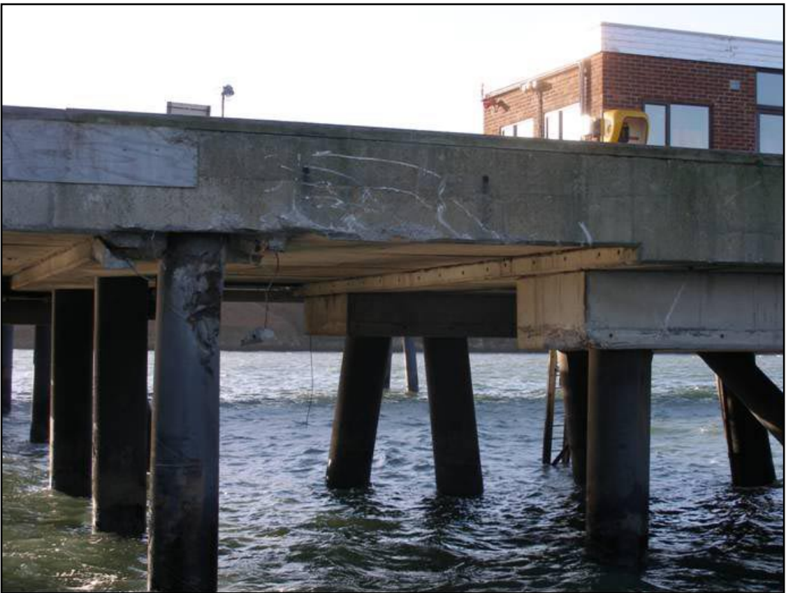
Damage to berth
