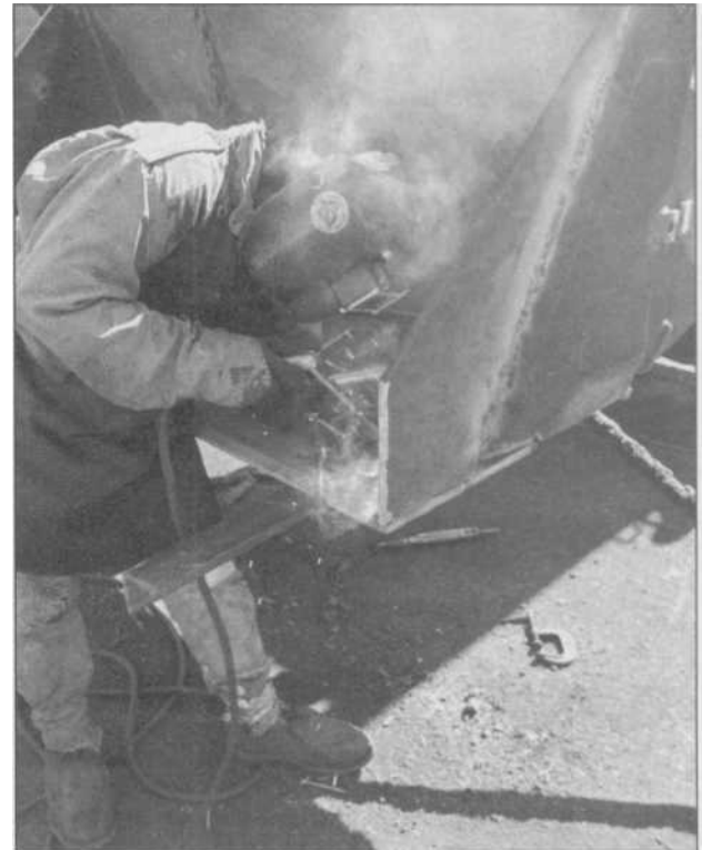
1.6 The construction and repair of heavy equipment and farm machinery would be nearly impossible without welding. Arc welding is usually used, as here modifying the front of a dirt scoop on a John Deere, where welding is outdoors and on heavy plates.
