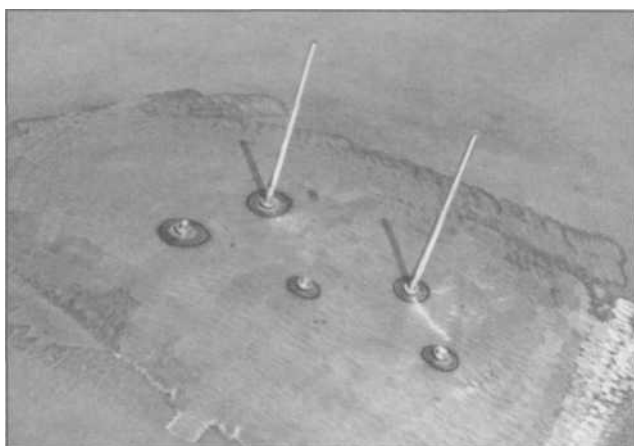
8.37 On this dent, the first three studs pulled out the bulk of the damage, and two more are in place to pull the last bit out. Note how the first three studs have been clipped off with cutting pliers.
