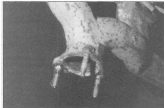
5.28 The new stud is now welded in place, with strength said to be up to 85% as good as original. This feature is a real time-saver for busy muffler businesses.
