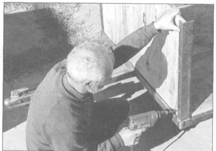
9.29 The front panel is attached with carriage bolts through the angle-iron posts. The posts were pre-drilled before welding on, because they are much easier to drill in a drill-press than once they are welded in place.
