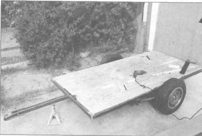
9.25 In our case, the frame was built just the right size to use an uncut 4x8-foot piece of 3/4-inch plywood for the trailer's floor.
