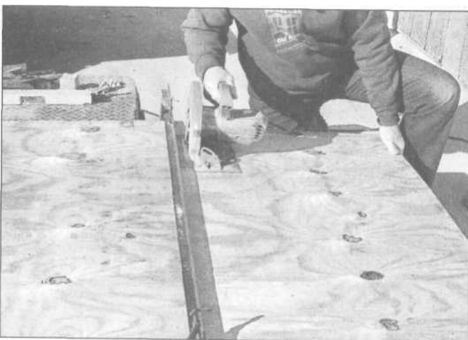
9.28 Having metal around for welding projects can pay off when working with wood, too. Use an extra length of straight angle-iron or tubing to clamp down on a piece of plywood as a saw guide, for perfectly straight cuts.
