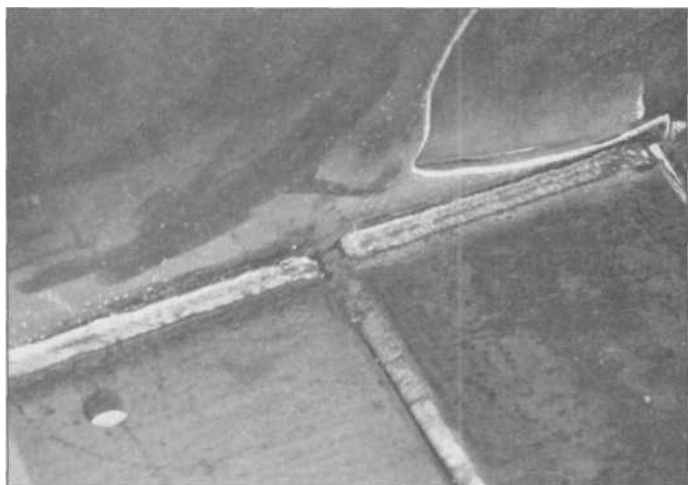
4.22 Here half-inch plate on the sides was welded with one pass, but a gap was left where the one-inch, beveled lower plates join. The bigger plate will be welded with several passes and strength is improved if the joint starts all the way at the ends.
