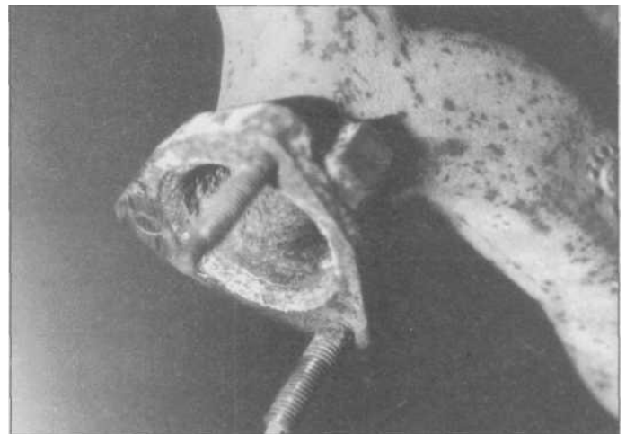
5.26 In exhaust system work, muffler shops deal with broken and rusted-away manifold studs all the time. HTP has a special feature to their MIG 160 that repairs such problems. First the old stud is cut off flush.
