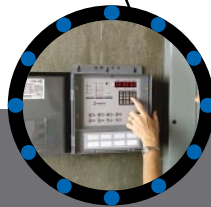
Whole home energy controls
