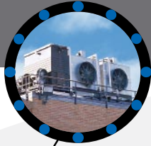
HVAC energy controls
