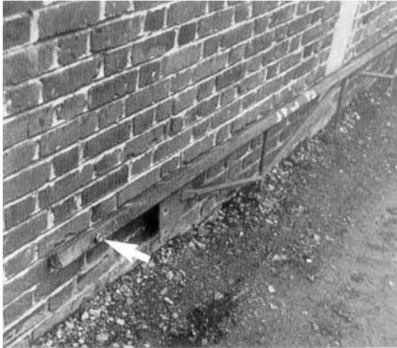
Figure 39: End of a lattice purlin with a bolt hole through the chord.
