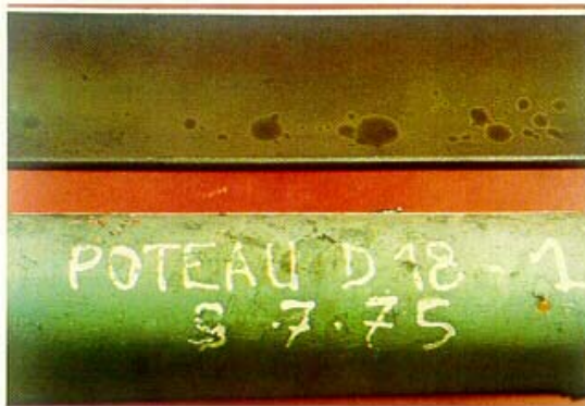
Figure 59: Tube with ends welded to the wall of another tube (Second inspection programme)
