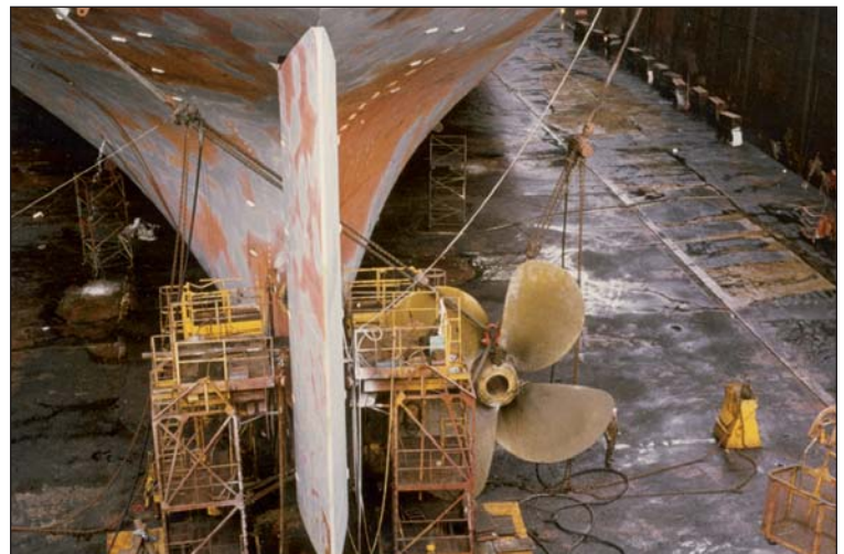
Concentrated power with sensitive controls. The dismantling of the propeller was completed with several JDN air hoists PROFI 50 TI.
