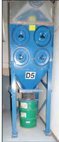
TORIT dust collector
