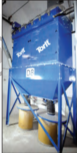
TORIT dust collector
