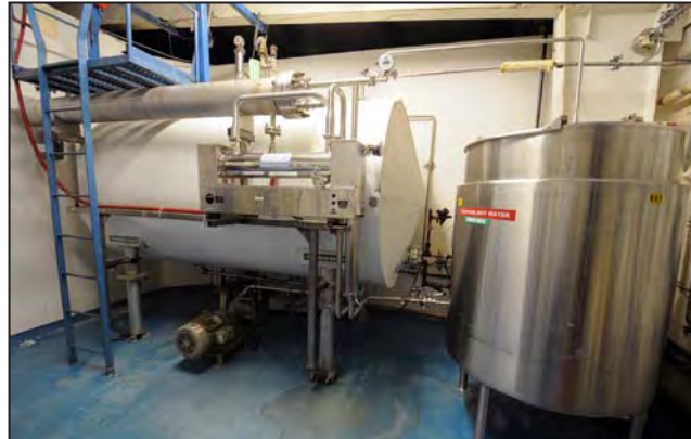
Water purification system
