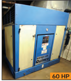
QUINCY air compressor
