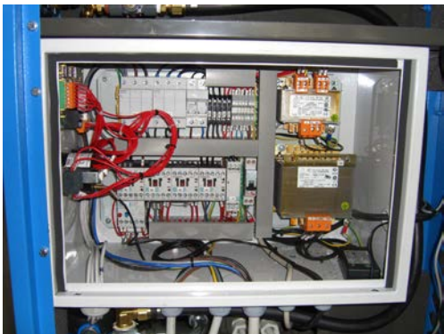
Electrical Box Located on right side behind panel.
