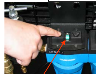
Differential Pressure Indicator Changes from Green to Red as Filter Ages. Do Not Use When Red.
