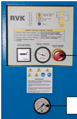
Emergency Shut Down Switch
