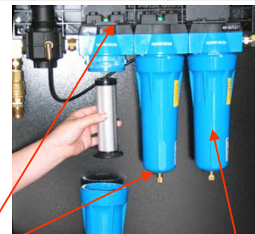
HF7 & HF5 Filters with Auto-Drain Floats & Differential Pressure Indicators.
