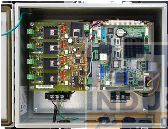
Figure 5-6 ePC with MHM in Remote Cabinet
