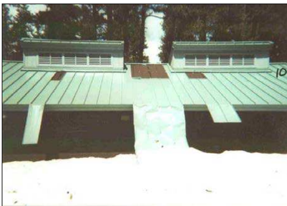
Figure 7-9 Adverse Effects of Snow Load on a Metal Roof
