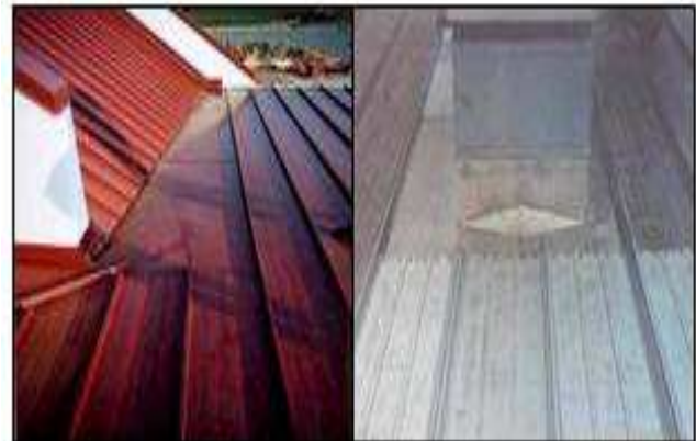
Figure 10-42 Proper Planning and Installation Avoids Ponding Issues
