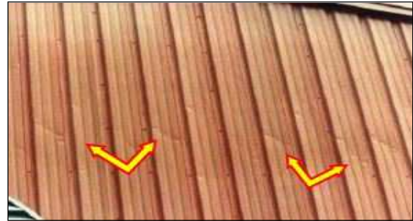
Figure 17-1 Carelessness During the Roof Installation Can Damage the Structure Siding
