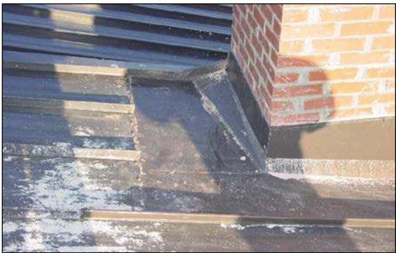
Figure 3-14 Roof Staining and Corrosion Caused By Wet Mortar
