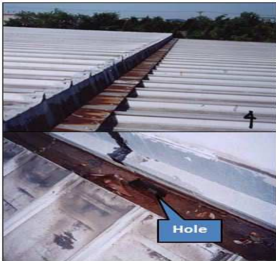
Figure 10-59 Incompatible Gutter, Flashing, and Roof Material
