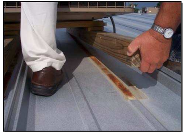
Figure 3-15 Roof Corrosion from Treated Wood
