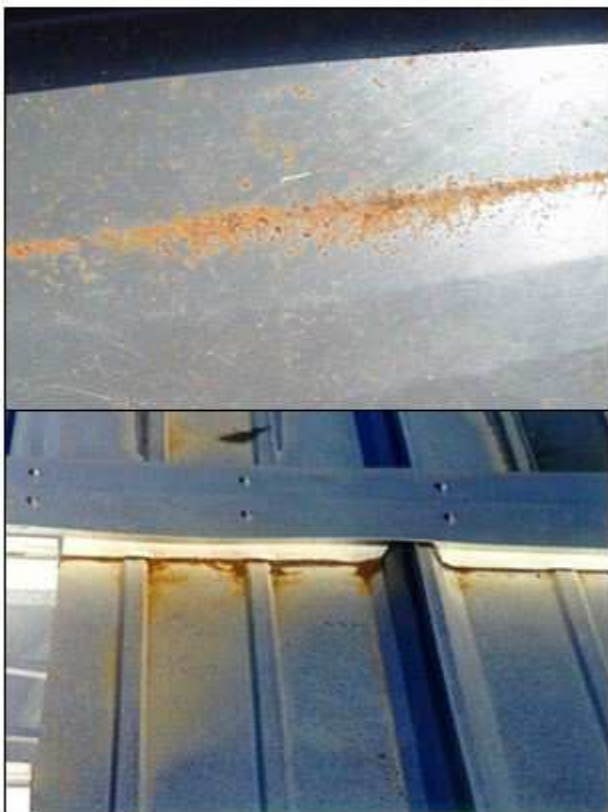
Figure 16-32 Failure to Remove Cutting Debris (Swarf) Quickly Causes Panel Corrosion and Rust
