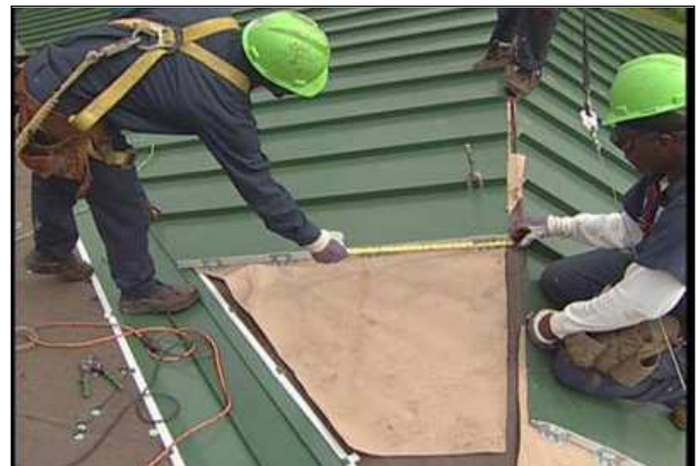
Figure 6-5 A Slip Sheet Is Often Installed Between the Underlayment and the Roof Panel.
