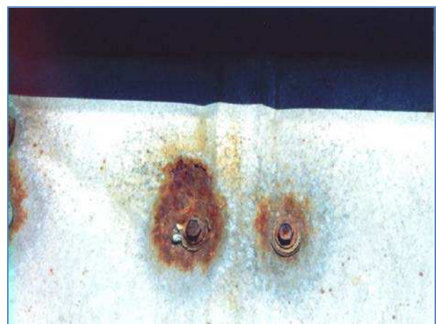
Figure 10-48 Incorrect Fastener Material
