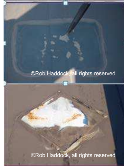
Figure 8-23 Failure of adhesive applied snow retention devices due to inadequate quantity, or design of system, or improper adhesive type, or bonding failure
