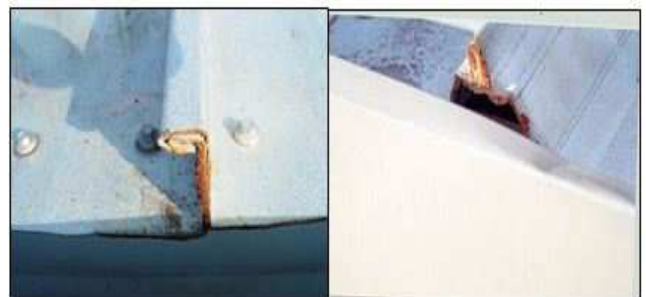
Figure 16-31 Premature Corrosion and Rust Due to Abrasive Cutting of the Panel
