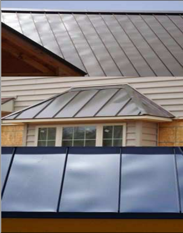
Figure 10-38 Oil Canning of a Metal Roof
