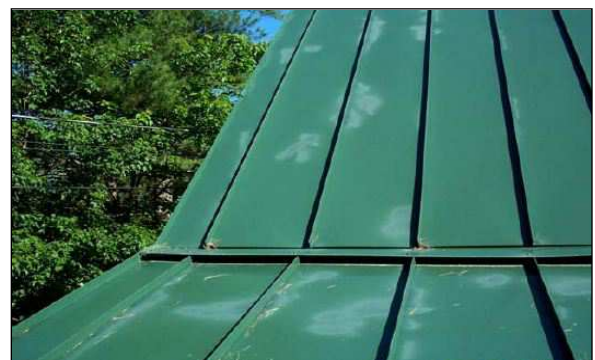
Figure 17-7 Touch-Up Paint Does Not Weather Like That of the Original Roof Panel
