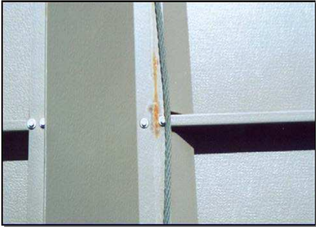
Figure 3-13 New Roof Corrosion from Direct Contact with Electrical Conductor
