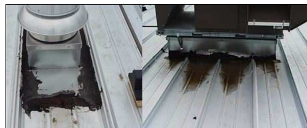
Figure 8-9 Improper Curb Types
