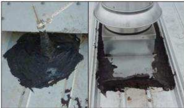
Figure 13-1 Old Methods and Materials Are Not Suitable In a Modern Installation
