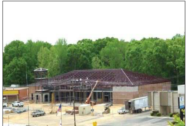
Figure 9-1 The Job Site Itself Presents Many Hazards
