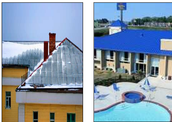
Figure 7-7 Temperature Extremes Are Normal for Any Roof
