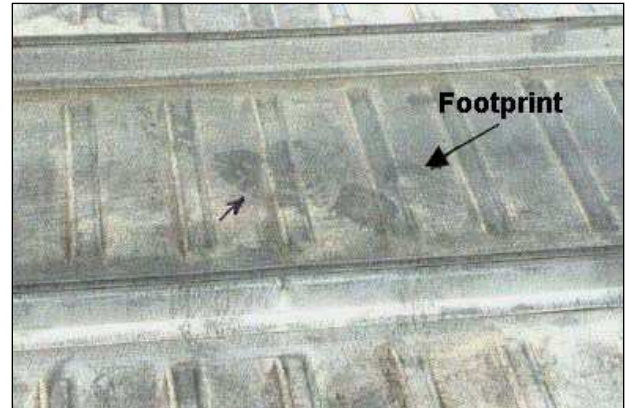
Figure 9-8 Inattention to Footwear May Cause Panel Damage
