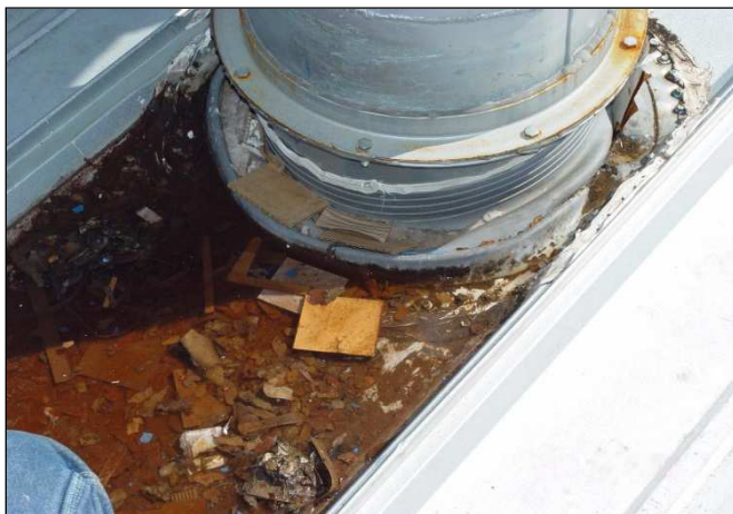
Figure 10-67 Improperly Installed Pipe Blocking Water Flow
