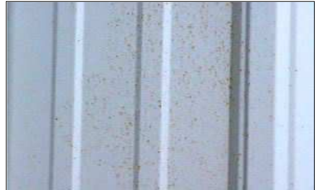
Figure 17-8 Panel Damage Resulting From Metal Filings Left On the Roof Surface
