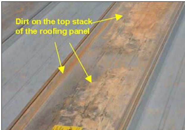
Figure 11-16 Uncovered, Stacked, Material Will Accumulate Significant Dirt on the Top Panel
