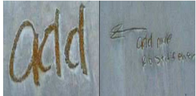
Figure 10-45 Corrosion Caused by Graphite Pencil
