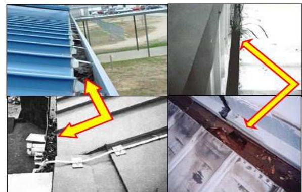
Figure 19-9 Gutters Need Cleaned and Inspected Regularly
