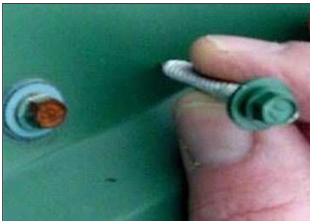
Figure 14-31 Correct Fastener Compared to Installed Fastener
