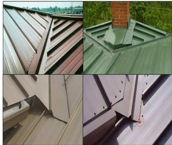
Figure 19-13 Valley Issues Affect Water Flow and Drainage
