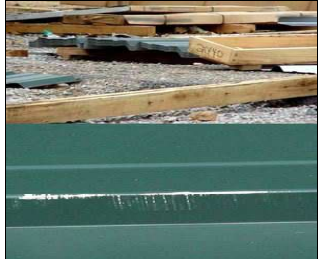
Figure 9-12 Improper Staging of Material Will Cause Damage
