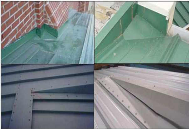
Figure 19-14 Roof to Wall Flashings Vary Widely
