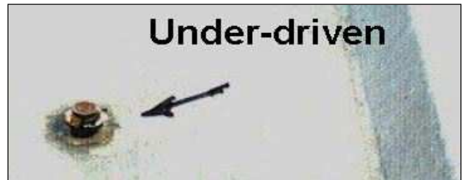
Figure 10-78 Under-Driven Fasteners Will Leak and Corrode
