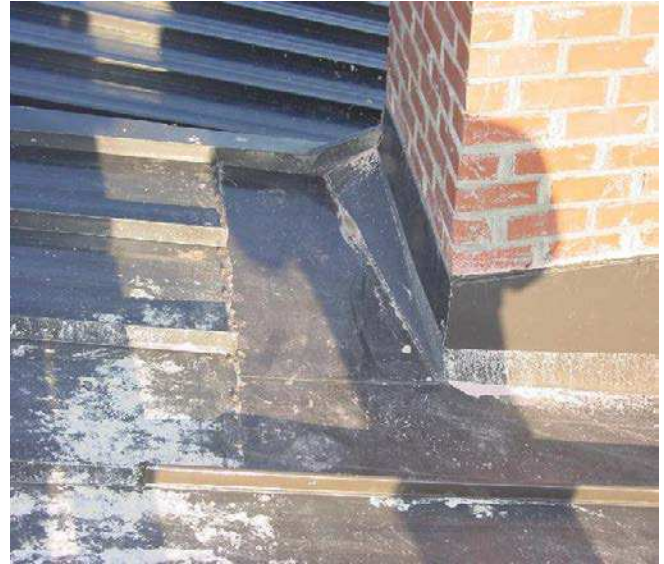
Figure 10-49 Cement, Mortar, and Related Products Can Damage Metal Roofs
