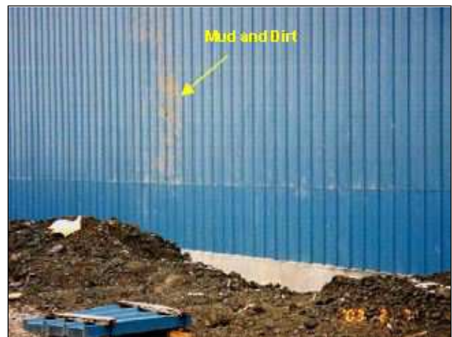
Figure 17-2 Spills and Runoff During Installation Often Affect the Structure Siding
