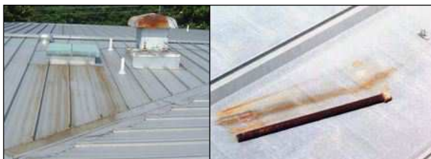
Figure 10-41 Corrosion Damage to a Metal Roof
