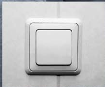
Light / irrigation controls
