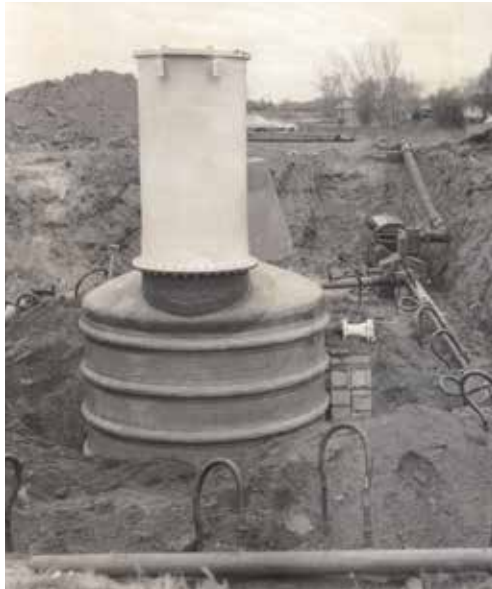
The first manufactured lift station by Gorman-Rupp was shipped to and installed in Hopkins, MN in 1967.
