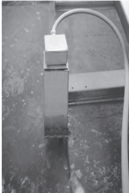
Electrode Probe installed in a Marley NC ® crossflow cooling tower
