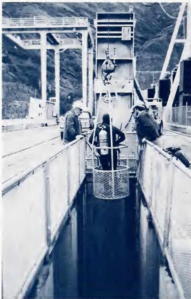
Figure 10-13 Diver Protected by Cage and Ready to be Lowered Into Dam Gatewell
