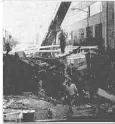
TOWER CRANE COLLAPSE (CLEANING UP DEBRIS)
