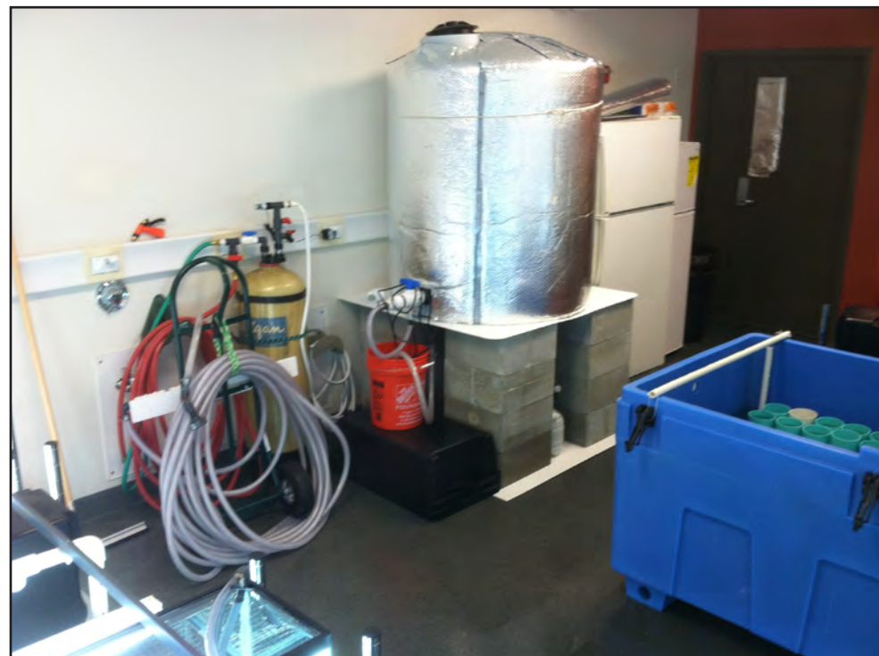
Figure 2.7 300-gallon holding tank and filtration system used in the nursery to fill the aquaria
