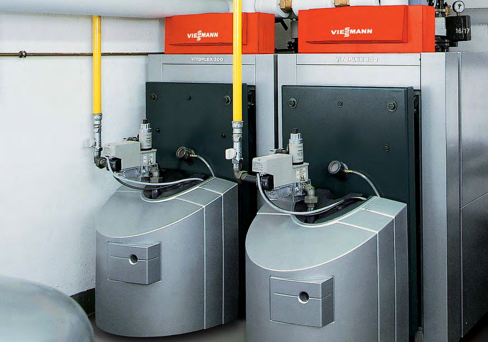
Heating centre with two Vitoplex 200 for output up to 1950 kW
