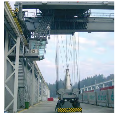
Spring cable reel Stock&Go on a spreader
