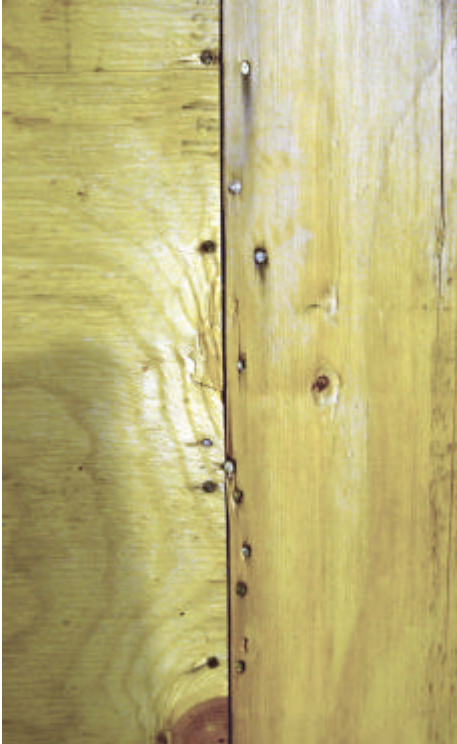
Fig. 3.46 Nails That Are Too Close to the Panel Edge and/or Overdriven
