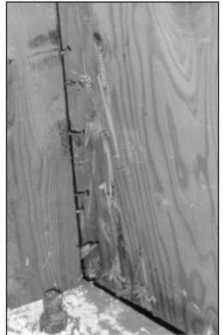
Fig. 3.45 Earthquake Damaged Shear Wall
