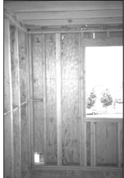
Fig. 3.28 - Too Far From Shear Wall End
