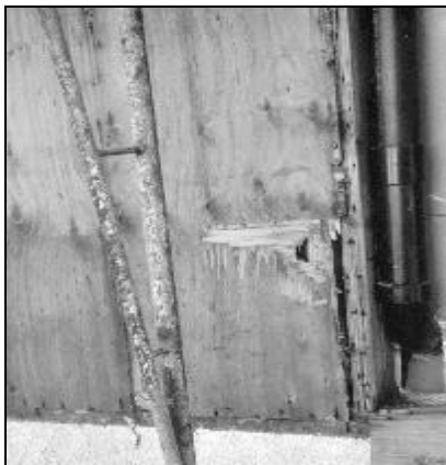
Fig 3.22 Earthquake damage with 2 inch adjoining stud
