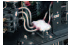
Coated Electrical Connections
