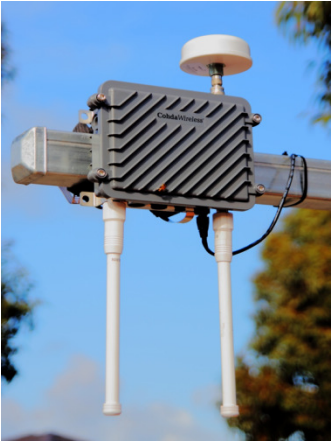
RSU attached to horizontal pole.
