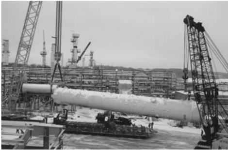
440 ton Gas Plant Vessel
