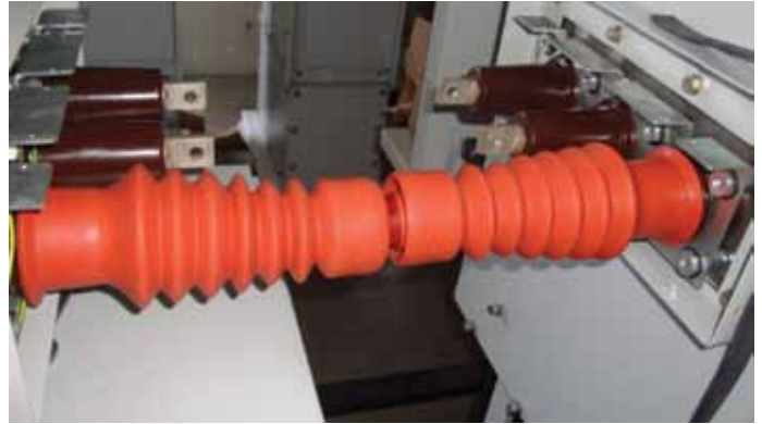
Sleeved busbars in coupled condition with insulating boot
