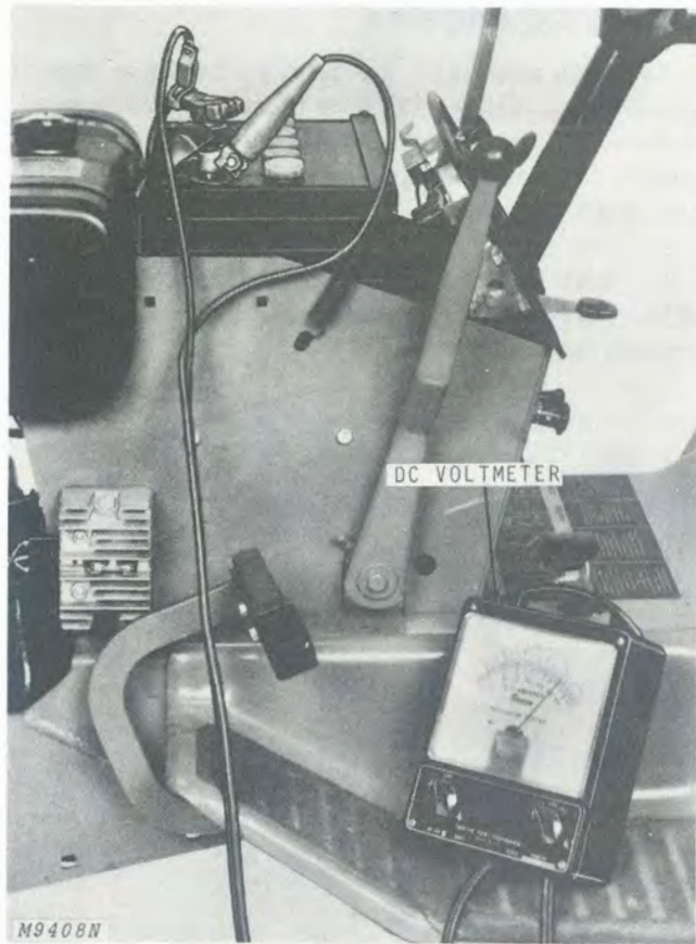
Fig. 10-Checking Battery and Regulator Condition
