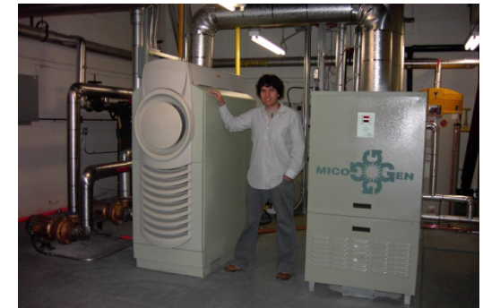
Microturbine CHP, Minto Hotel, Ottawa
