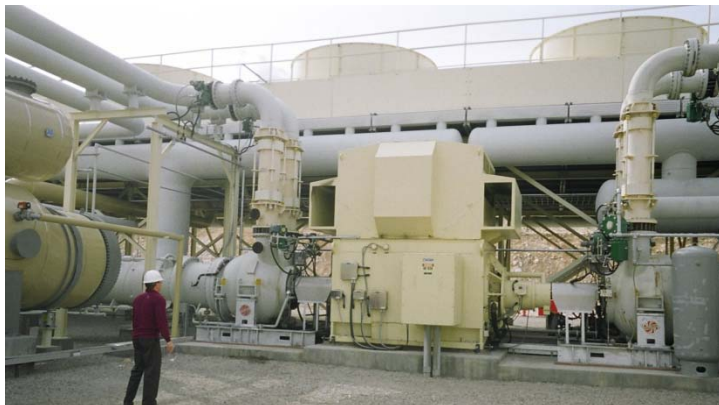
ORMAT Pentane Turbine Set
