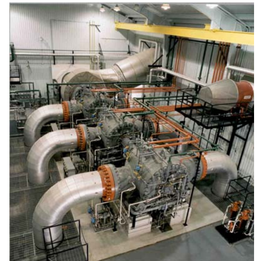
RB211 driven compressors, Union Gas Storage, Dawn ON
