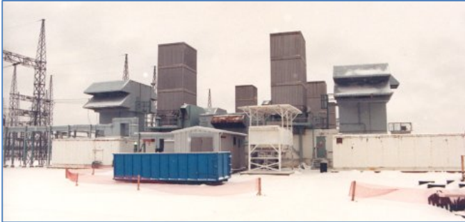
RR Olympus POD-50 units Cadillac Stn, Hydro Quebec
