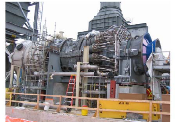
A close-up of the GE Fr7FB combustion turbine at Goreway
