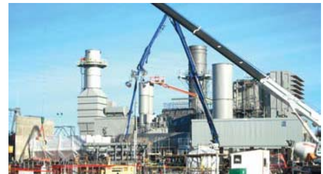
4 GE Fr7, Hydro Quebec Becancour, Gentilly Standby
