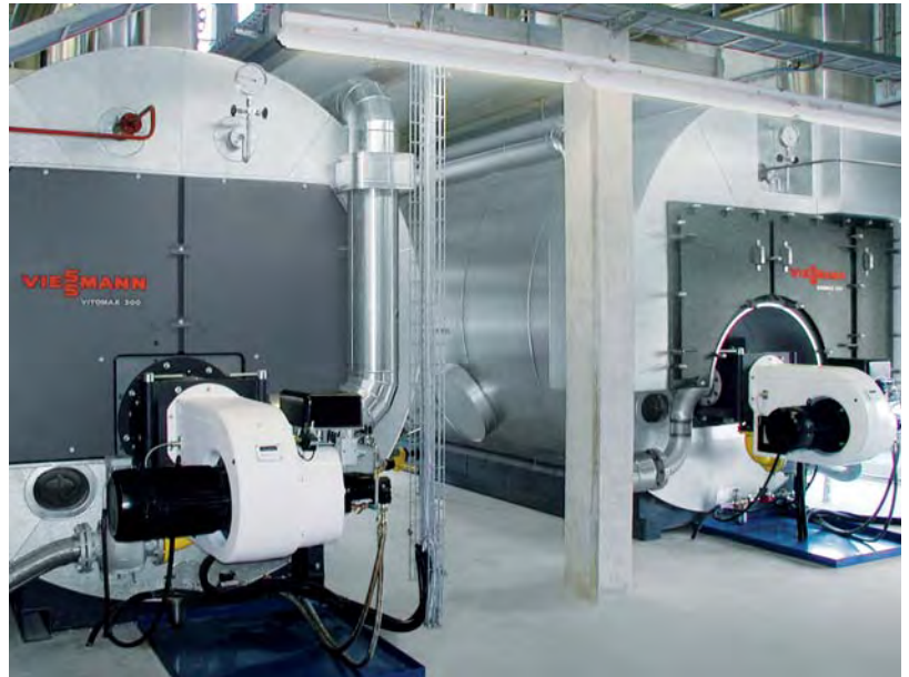
Steam boiler with waste heat utilisation combined with a conventional steam boiler
