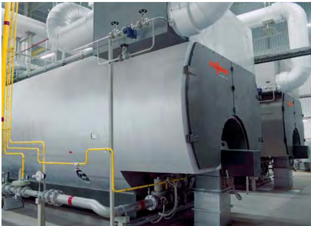
Steam boiler with superheater at Klaipėdos Kartonai, Lithuania
