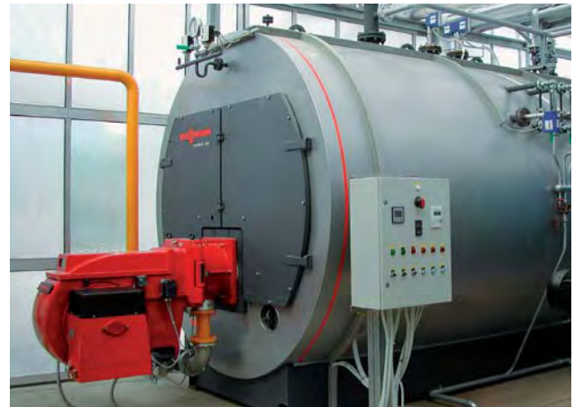
Vitomax 200-HS high pressure steam boiler in a commercial nursery
