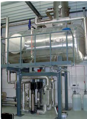
Feedwater tank with thermal deaeration
