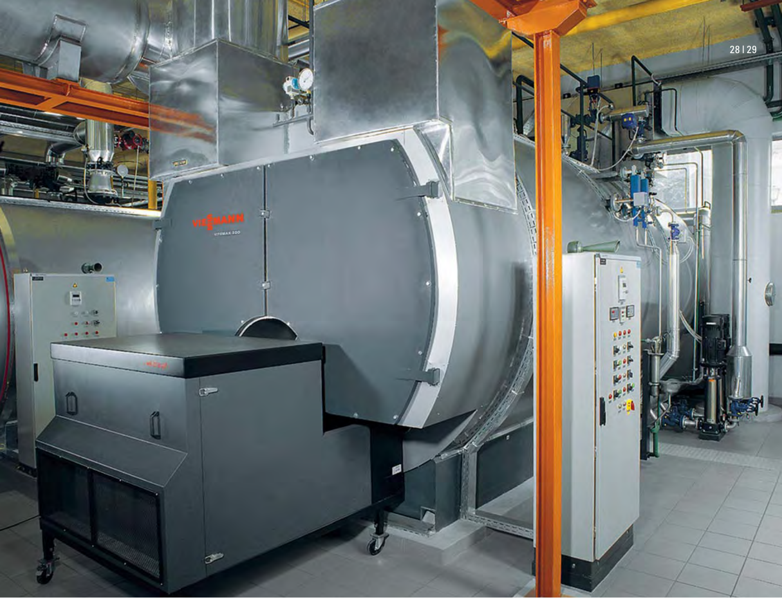
Vitomax 200-RS steam boiler with waste heat utilisation at the Maribor hospital, Slovenia (6 t/h, 13 bar saturated steam)
