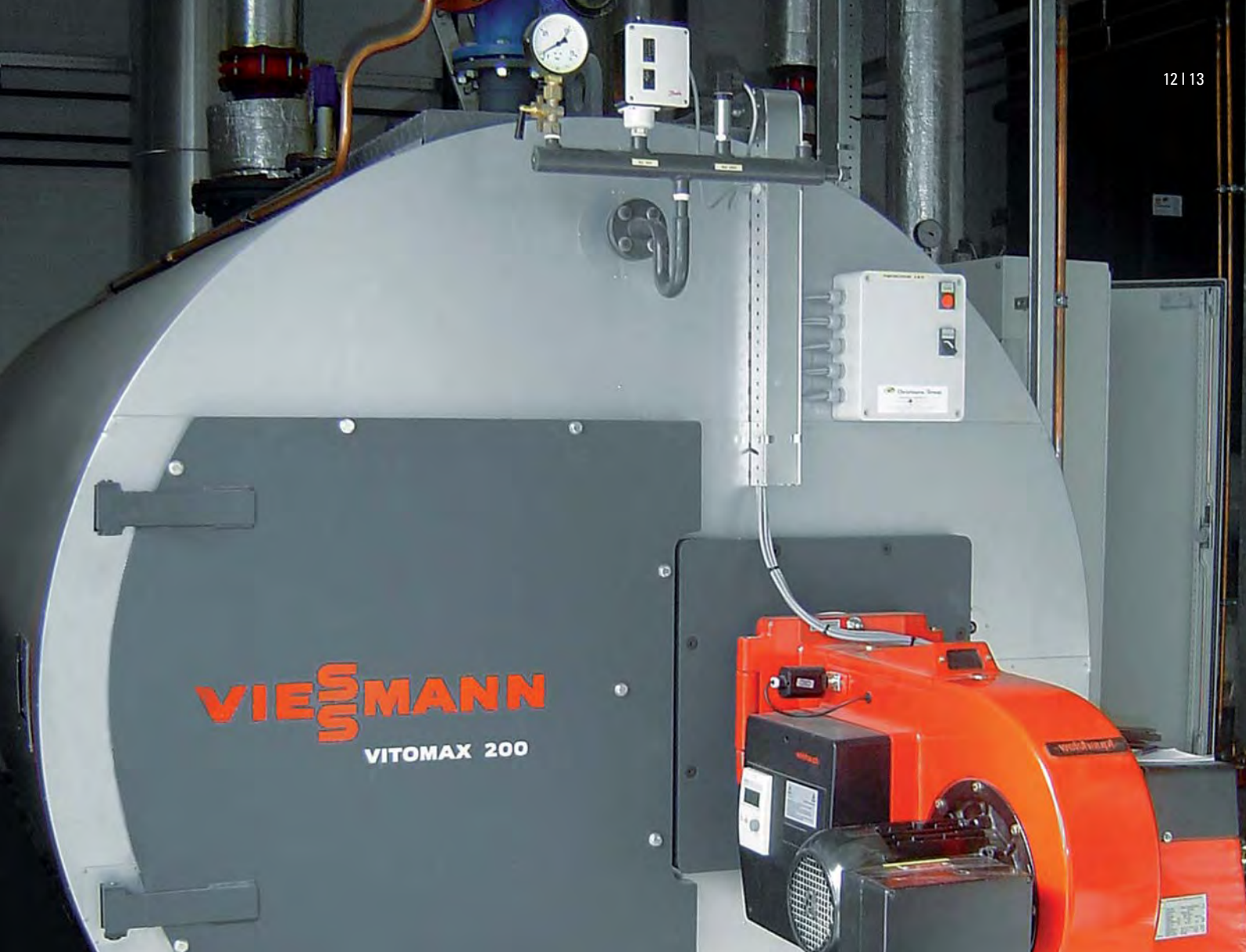
Vitomax 200-LS low pressure steam boiler Deckers Pilzen complex, Holland
