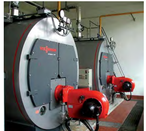
Steam boilers at the Rivolta Carmignani textile plant in Milan, Italy
