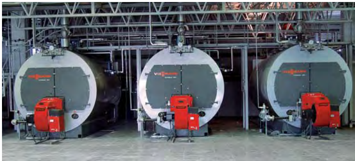
Steam boilers at Sanovel in Istanbul, Turkey
