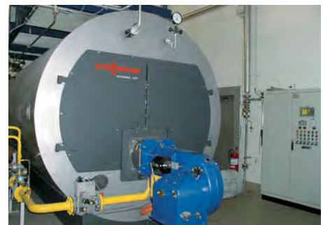
Steam boiler at AZM Asur, Belgium
