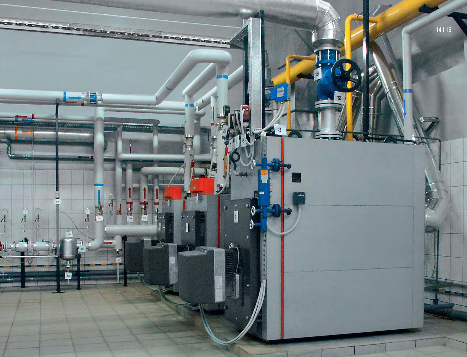
System with one Vitoplex 100-LS low pressure steam boiler and two Vitoplex hot water boilers
