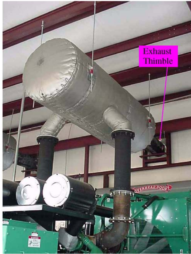
FIGURE 55. GENERATOR SET EXHAUST SYSTEM FEATURES. DUAL SIDE INLET SILENCER, FLEX CONNECTORS, EXHAUST THIMBLES, AND MOUNTING HANGERS ARE SHOWN.
