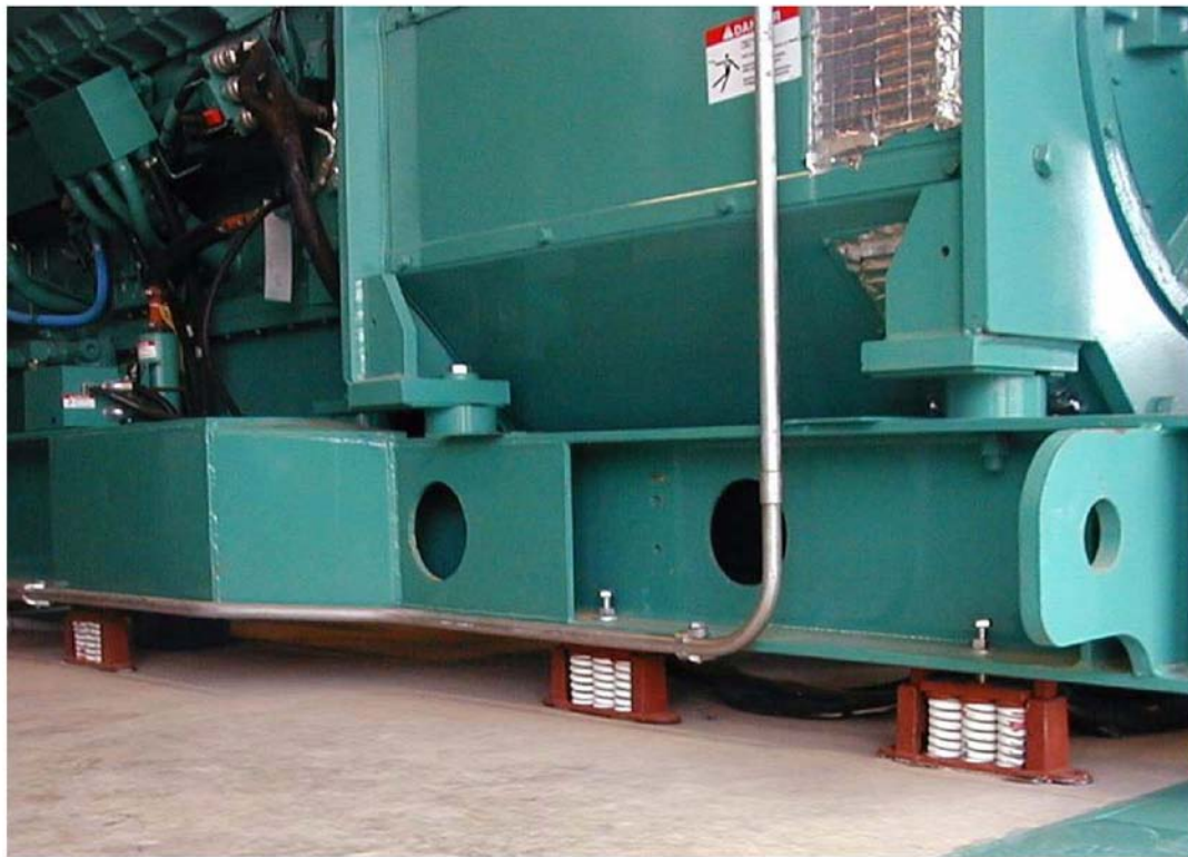
FIGURE 52. A GENERATOR SET MOUNTED WITH SPRING-TYPE VIBRATION ISOLATORS
