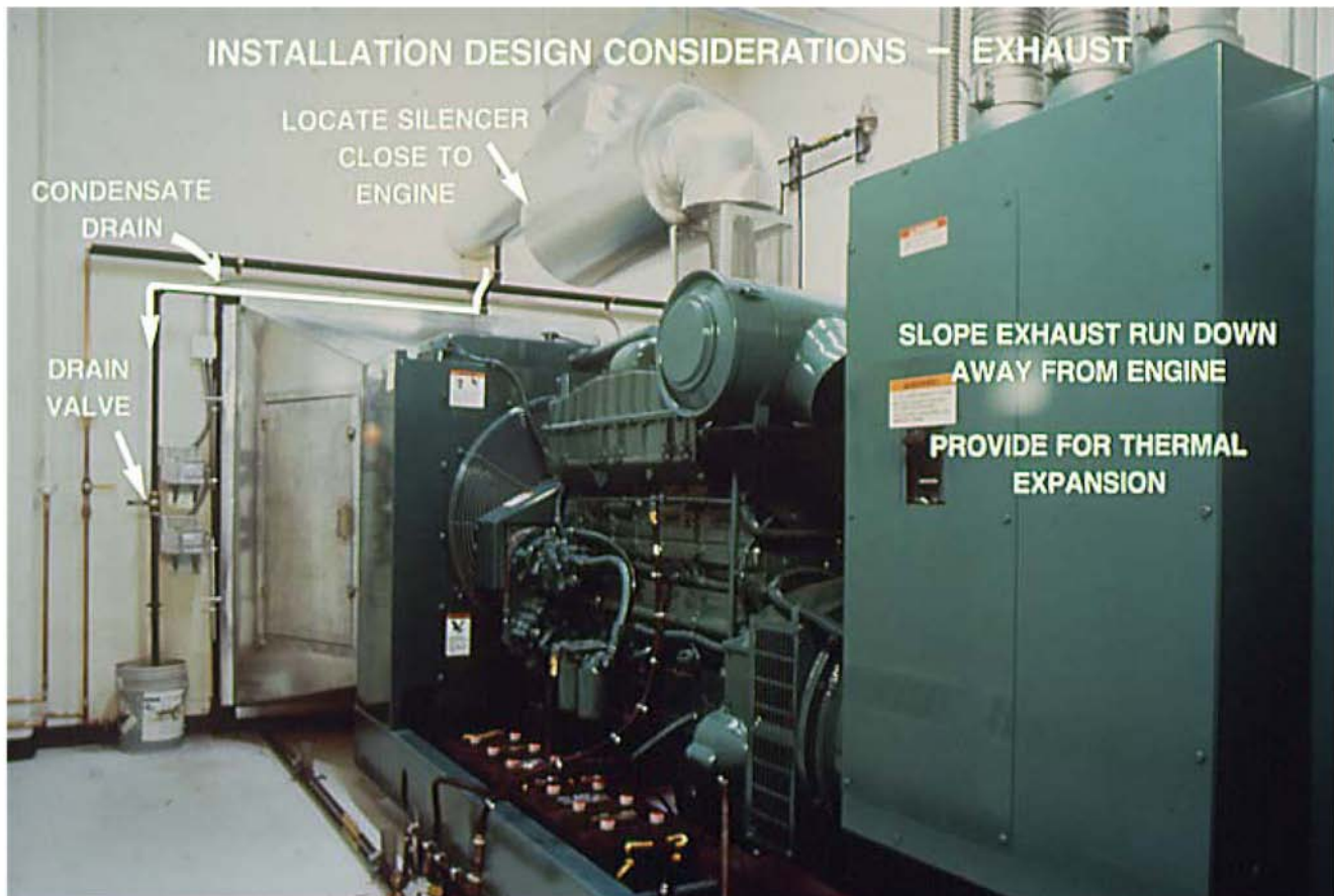
FIGURE 53. TYPICAL FEATURES OF AN EXHAUST SYSTEM FOR A GENERATOR INSTALLED INSIDE A BUILDING.
