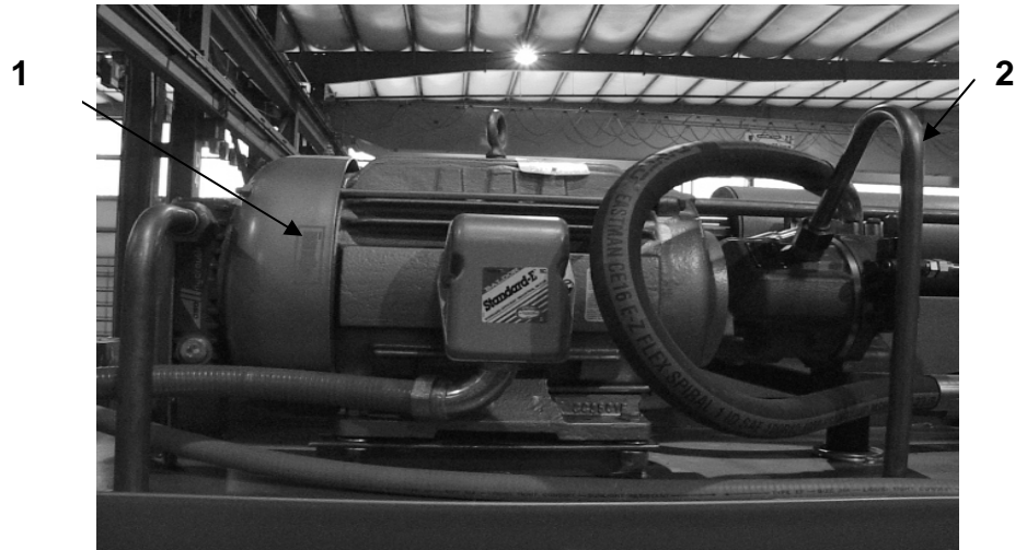
Figure 6: Hydraulic Pump/Motor Assembly Unit
