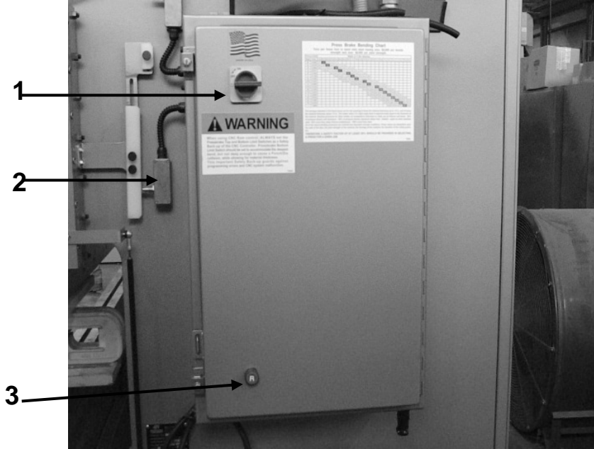
Figure 7: Main Electrical Enclosure
