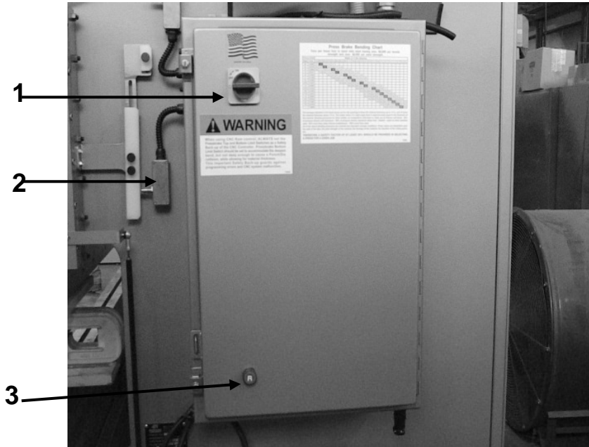
Figure 7: Main Electrical Enclosure
