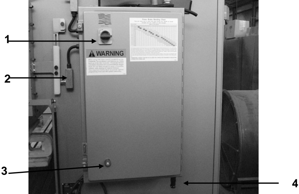
Figure 7: Main Control Panel
