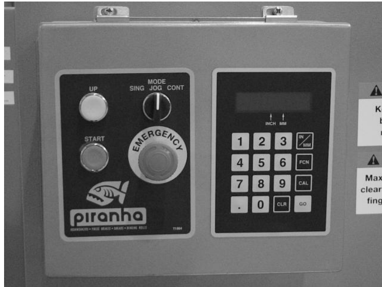
Figure 5: Main Control Panel-Programmable GOTO
