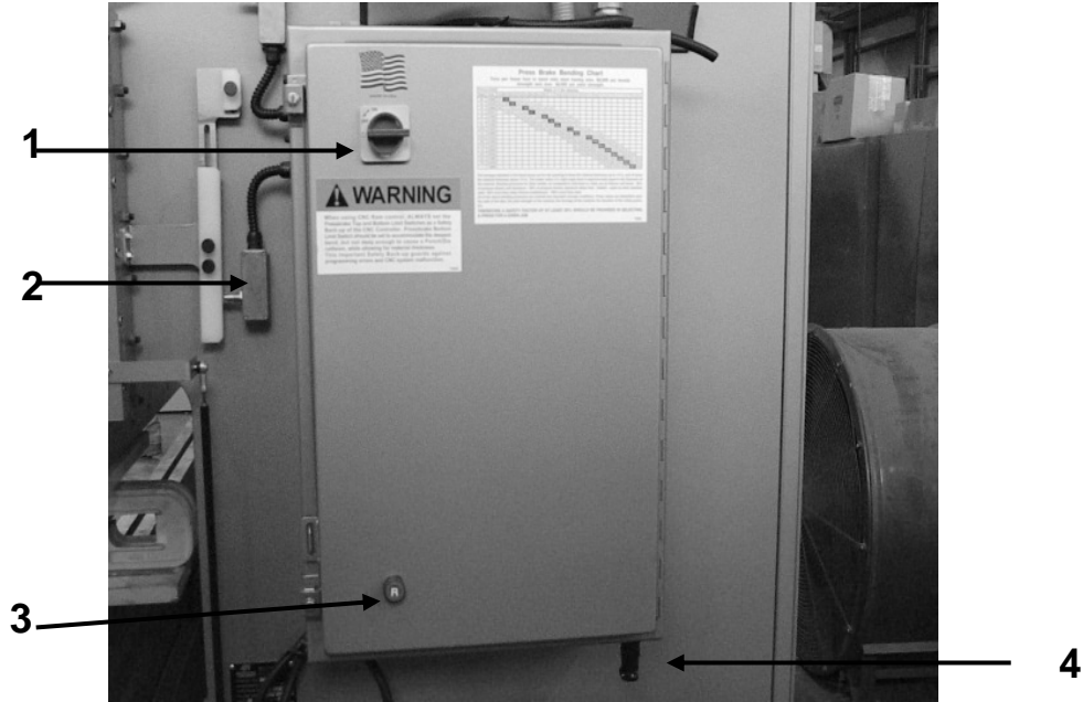
Figure 7: Main Electrical Enclosure
