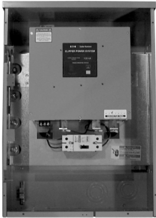
Group Metering — Surge Cubicle
