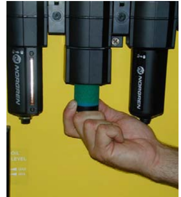
Changing LP Filtration Element
