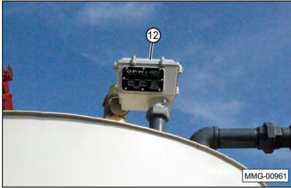
(12) Tank Level Gauge.
