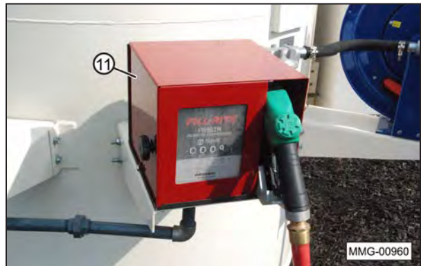
(11) Fuel Dispenser and Meter.
