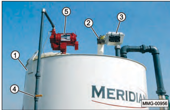
(1) Fuel Tank. (2) Tank Vent. (3) Tank Level Gauge. (4) Fuel Shutoff Valve. (5) Top Mounted fuel pump.
