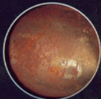
Actual photo taken through Lenox sectional borescope showing corrosion deep inside long section of pipe
