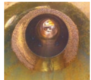
rust and corrosion in downstream section without proprietary internal coating after only six months in use
