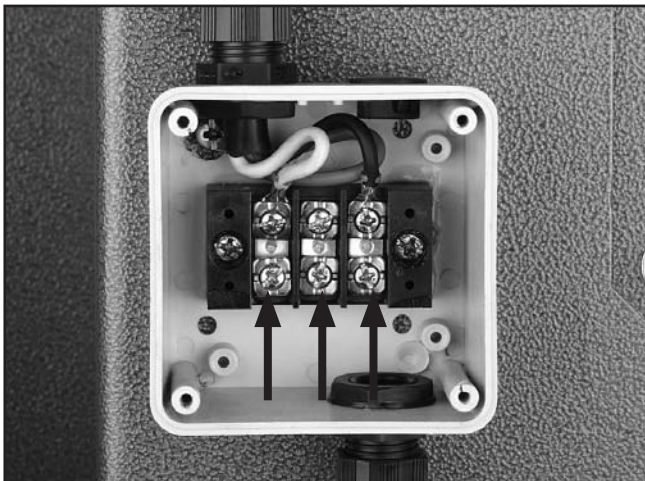
Figure 47. G0591 main terminal box.
