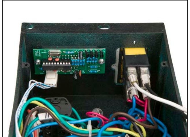
Figure 96. Control panel wiring (top).
