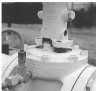
PACKING GLAND BOLTS EXPOSED
