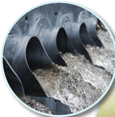
A sewage water treatment plant
