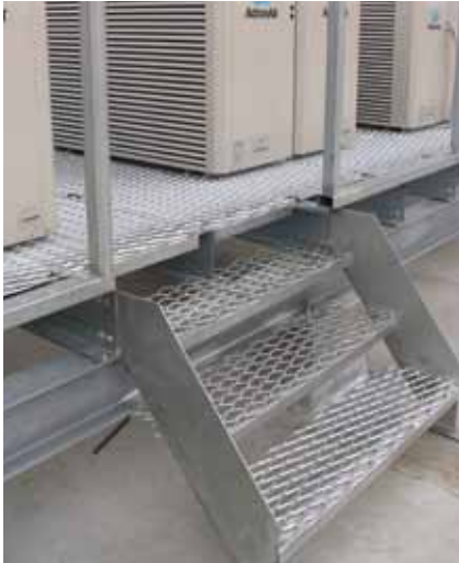
Air conditioning platforms
