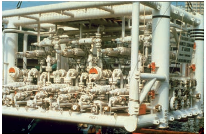
MOV chokes within a offshore platform installation.
