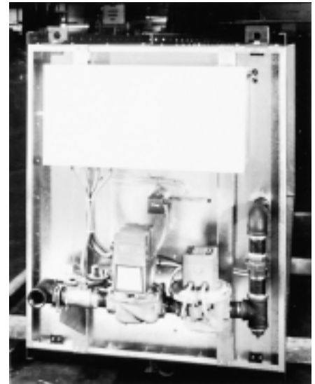
Gas manifold and control cabinet
