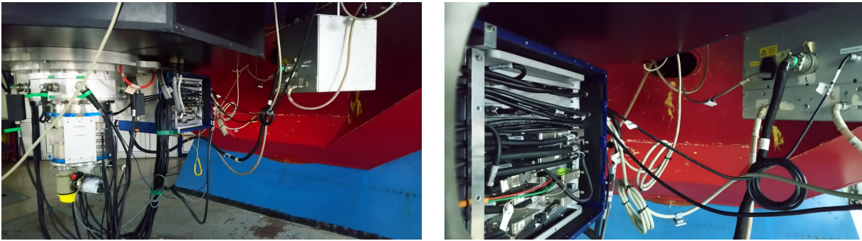
Figure 9.5: WFI electronics. The box on the right controls the power and can be used to power cycle. The box on the left contains the electronics boards that one may need to unplug and replug.
