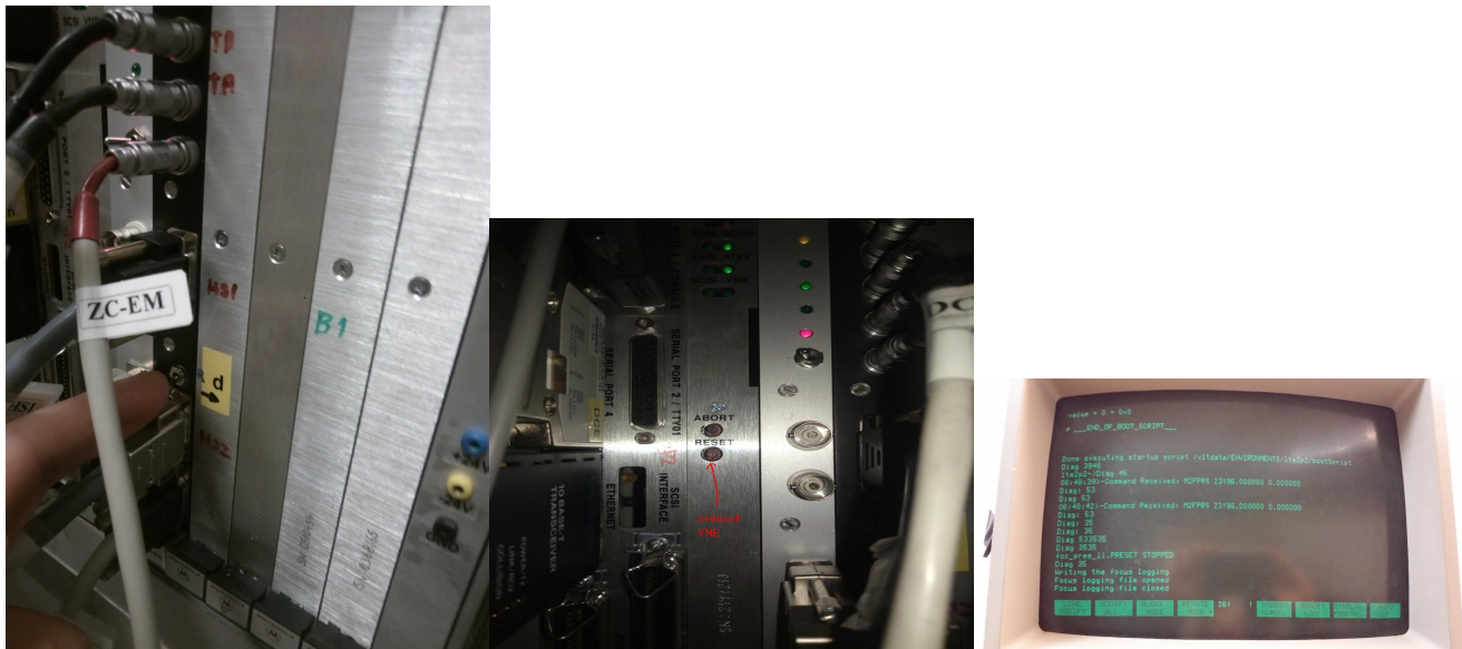
(a) Remote/local pointing control
