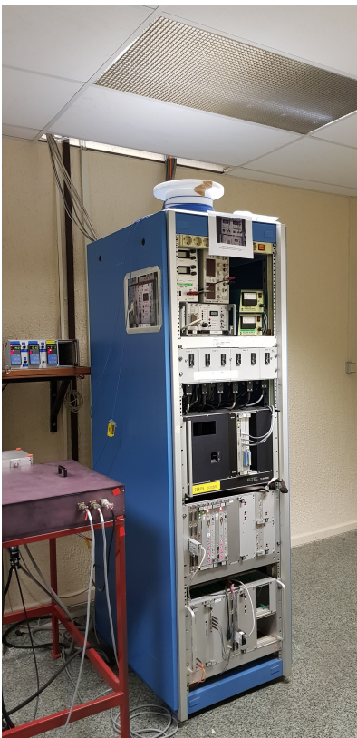
(a) Rack tower
