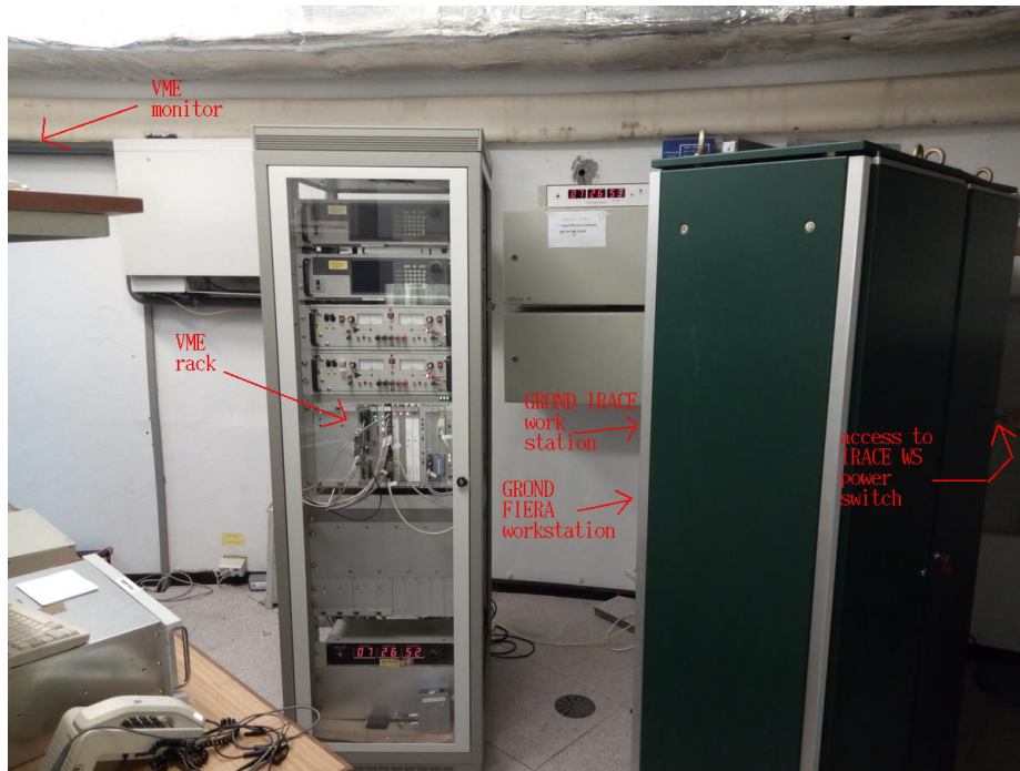
Figure 1.4: Entering the computer room in the telescope building. In front slightly to the left is the VME rack.
