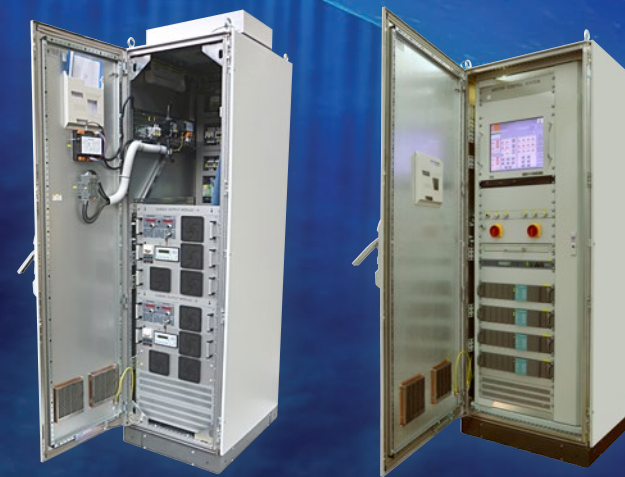
Electrical power unit.
