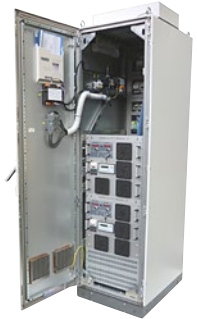
Electrical power unit.
