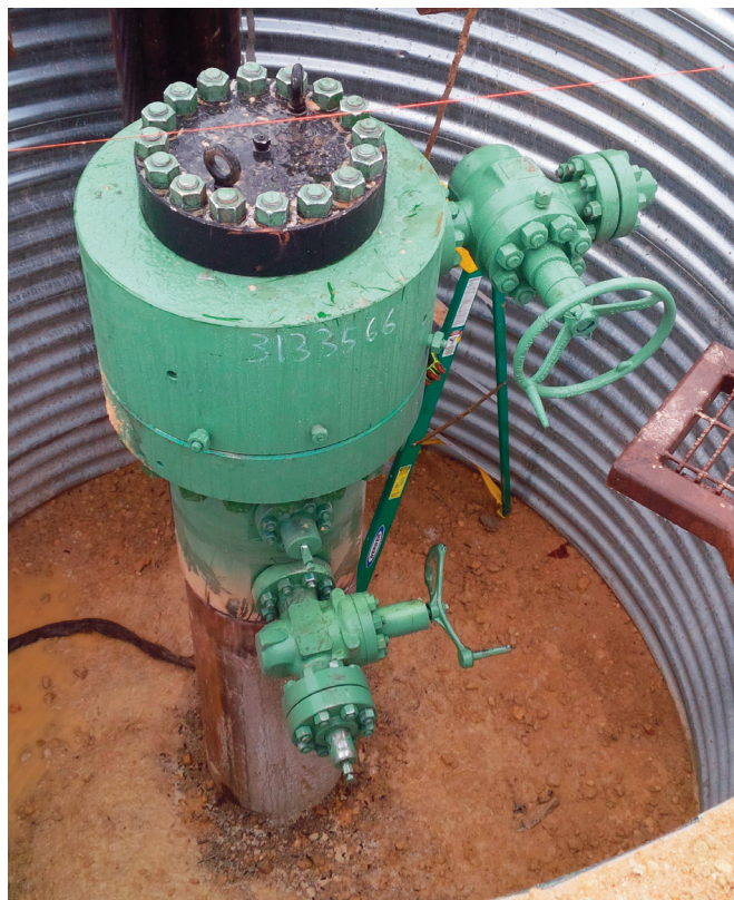
Figure 3. An example of advances made in the area of wellhead reliability and functionality for unconventional is Cameron's advanced multi-bowl nested diverter snap ring (MN-DS) wellhead system.
