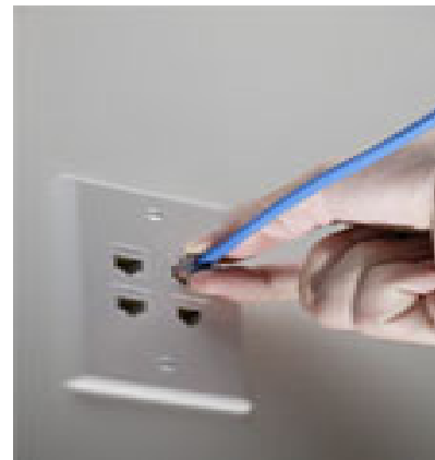
Wall Data Port
