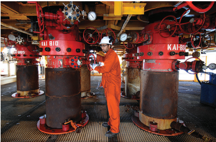
A qualified Cameron technician monitors wellhead performance.
