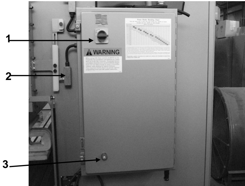
Figure 6: Main Electrical Enclosure
