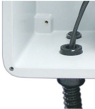
Figure 7-2 Protective Armored Conduit and NPT Fitting on the STS Enclosure
